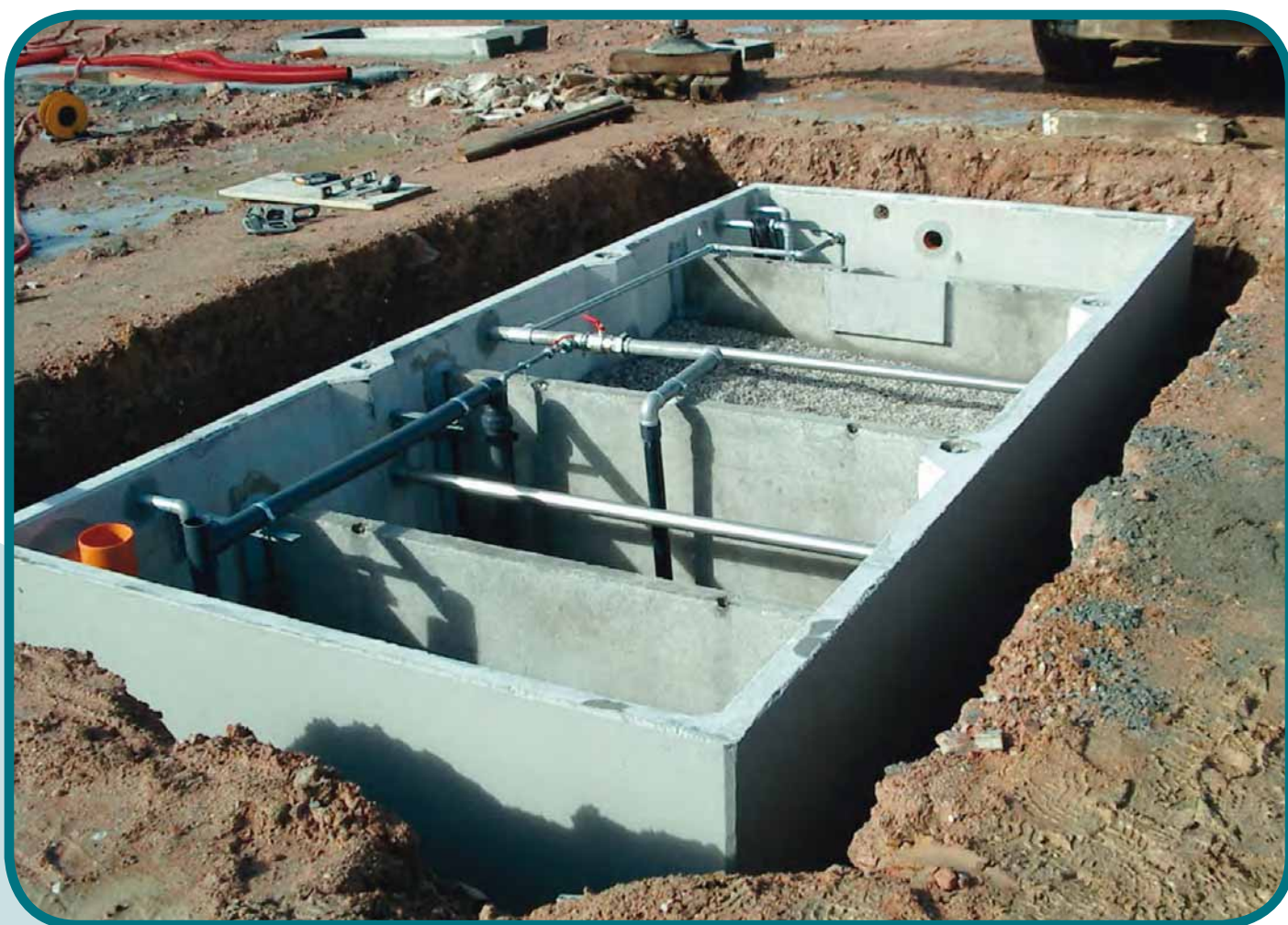
Vista parte interrata depuratore 4F/P Prefabricated underground tank of 4F/P wastewater treatment plant
