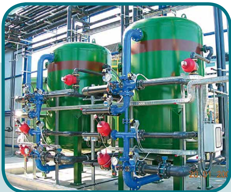
Filtrazione su resine chelanti per metalli – Portata 50 m 3 /ora Chelating resins for metals filtration system – Flow rate 50 m 3 /h
